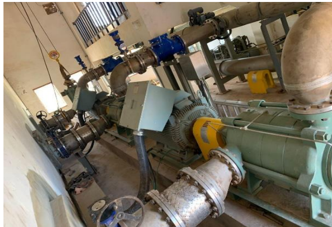
Rehabilitated pumps at Jabusie Headworks – UWR
