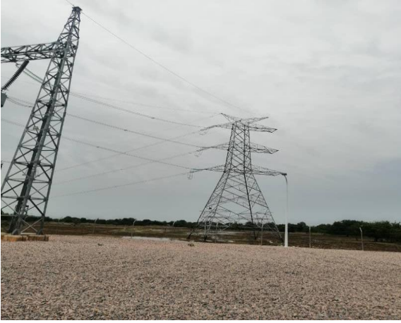
330 kV Kumasi-Kintampo- Navrongo Line
