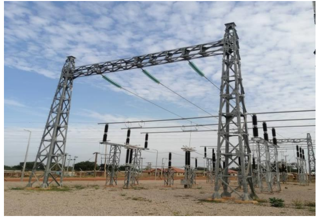
Tamale- Bolgatanga 161kV Line upgrade
