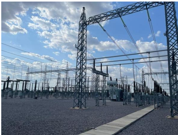
Kintampo – Adubiyilli 330kV Line
