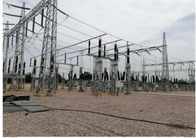
330 kV Kumasi-Kintampo- Navrongo Line
